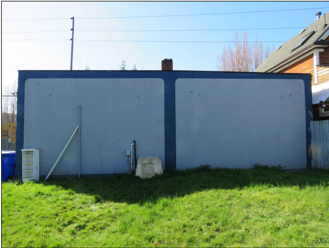
Photograph 9 of 22: OR_MultnomahCounty_DeansBeautySalonandBarberShop_0009 View of rear (north) façade and backyard, camera facing south.
