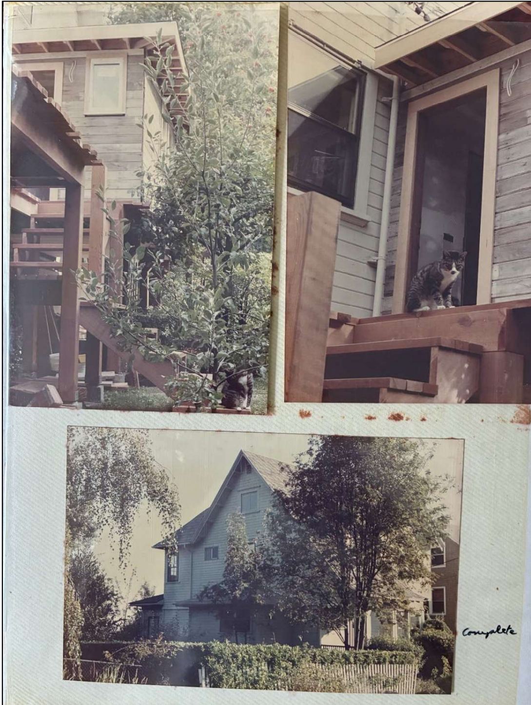
Figure 13: Construction photos showing 1984 Laundry Room Addition. Views looking at west elevation. Source: Le Guin Family Collection.
