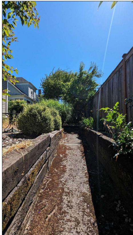
Photograph 6 of 15: OR_MultnomahCounty_JuniperHouse_0006 Concrete ramp on the south of the lot. Camera facing east.
