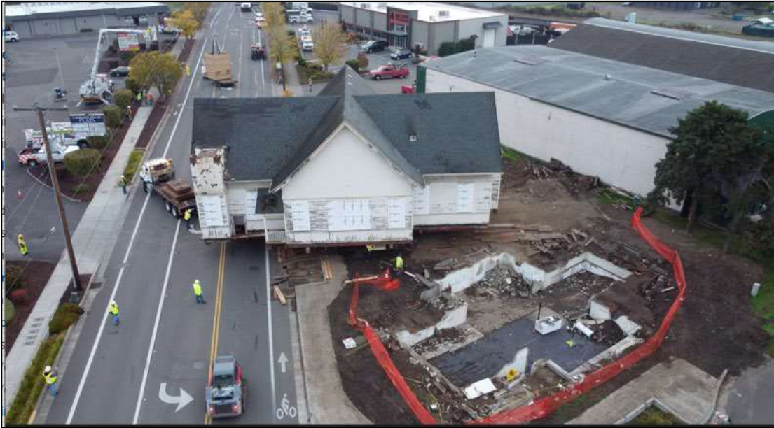
Figure 20: Image of Cumberland Presbyterian Church being moved off foundation and onto Santiam Road
