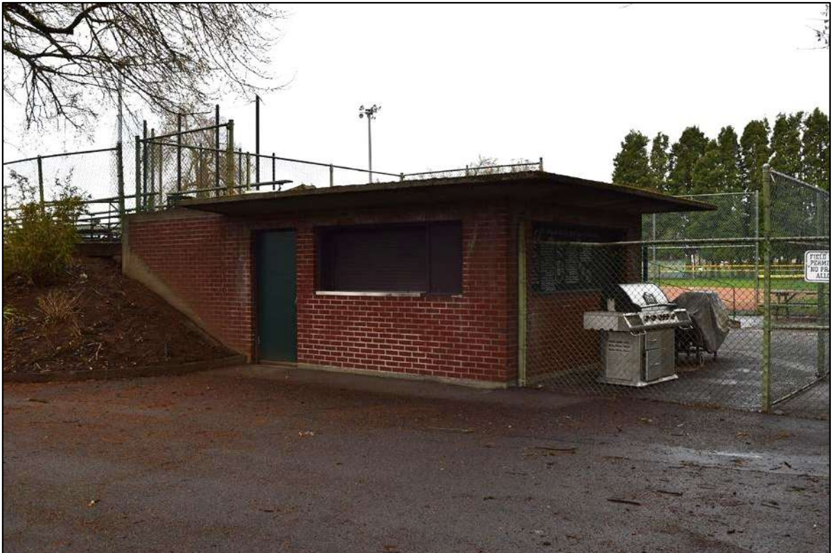
Photo 4 of 14: OR_Multnomah_NormandaleField_0004 Looking southwest at the concessions building from the east field sidewalk frontage
