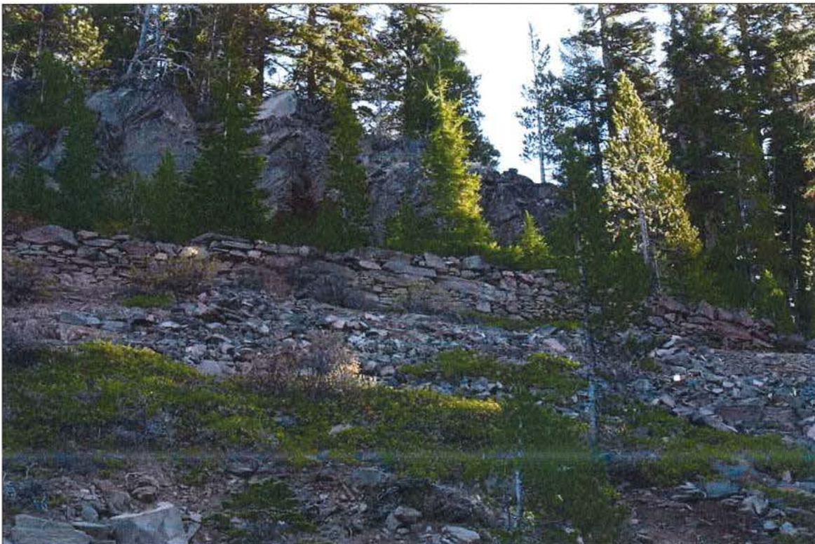
Photo 18 of 20: Rim Road revetment (retaining wall) at center, located between Kerr Notch and Anderson Point, looking east
