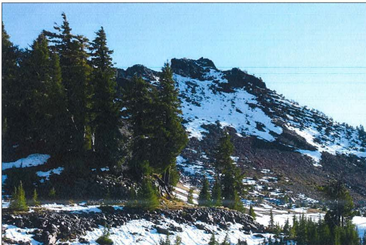
Photo 6 of 20: Part of Rim Road revetment in left foreground near Hillman Peak, looking south
