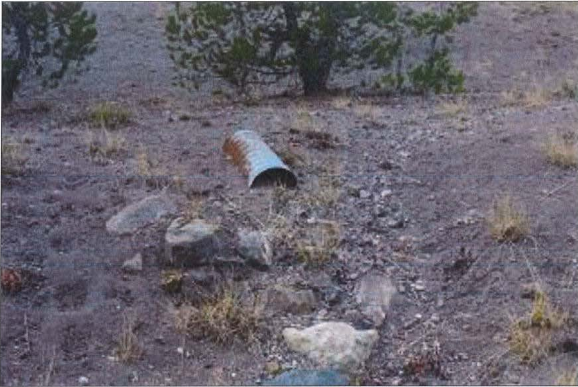
Photo 17 of 20: Section of abandoned Rim Road showing metal culvert and cross drainage failure, looking west
