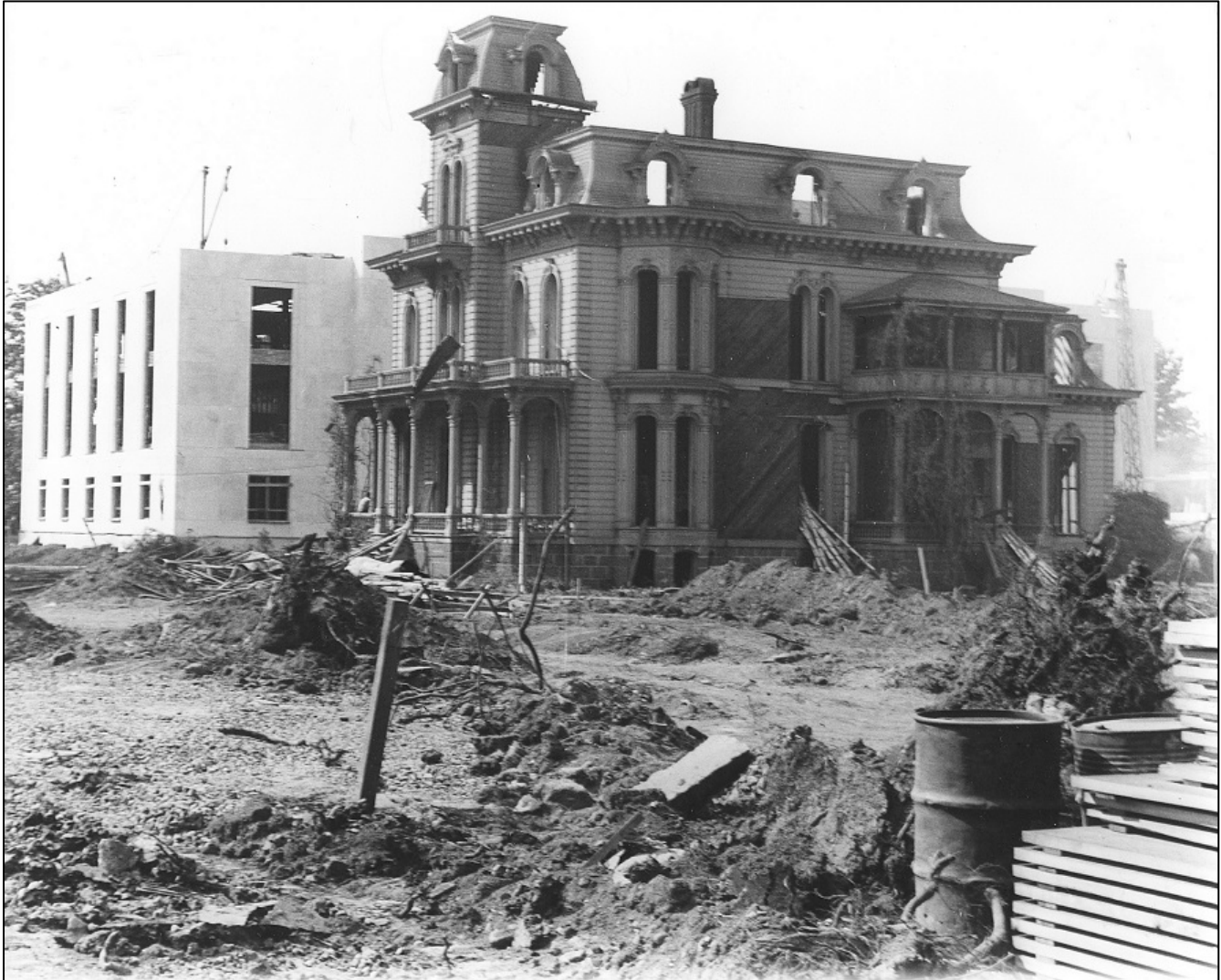
Figure 14 – View of Block 83 from southeast, September, 1938. View of Cooke-Patton house in front of east elevation of library, prior to demolition of house.
