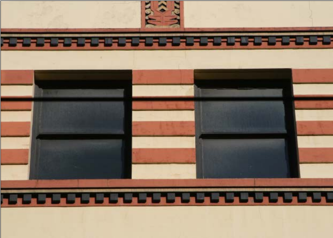
Photo 7 of 14: Exterior Detail, east elevation, looking west, decorative Zig-Zag trim at fifth floor (typical)
