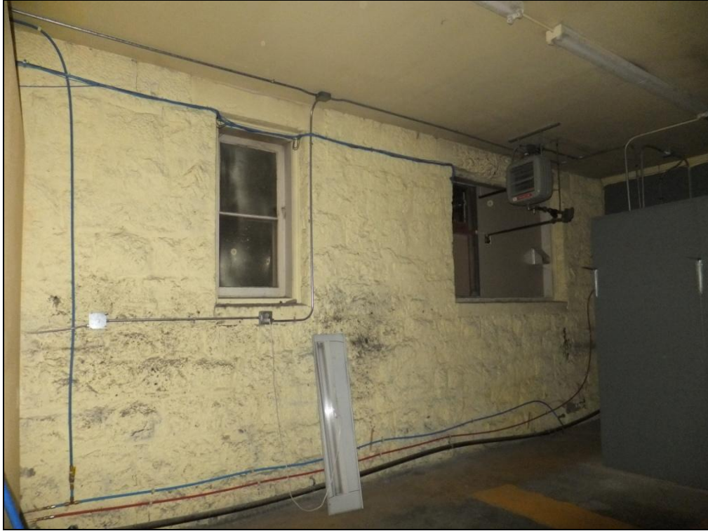
Photo 9 of 11: OR_WallowaCounty_WallowaCoChieftainBuilding_0009 New Press Room, looking south to the original outer wall of the Wallowa County Chieftain Building
