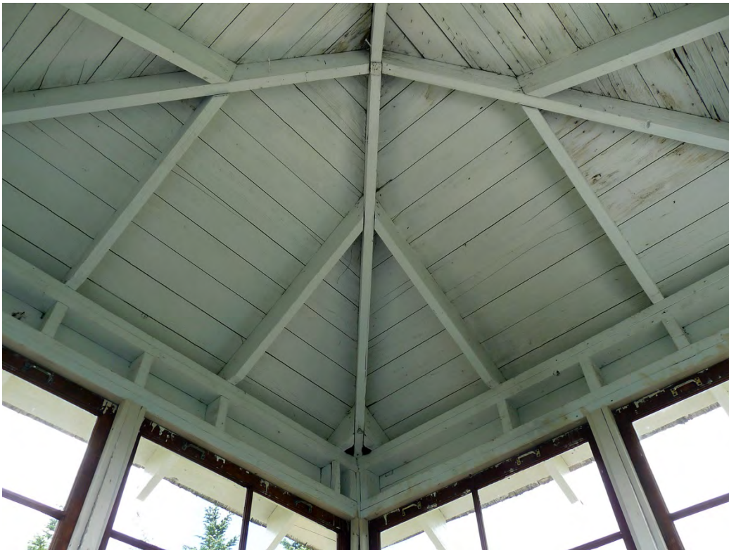
Figure 11. View of the construction of the interior of the roof in the cupola.
