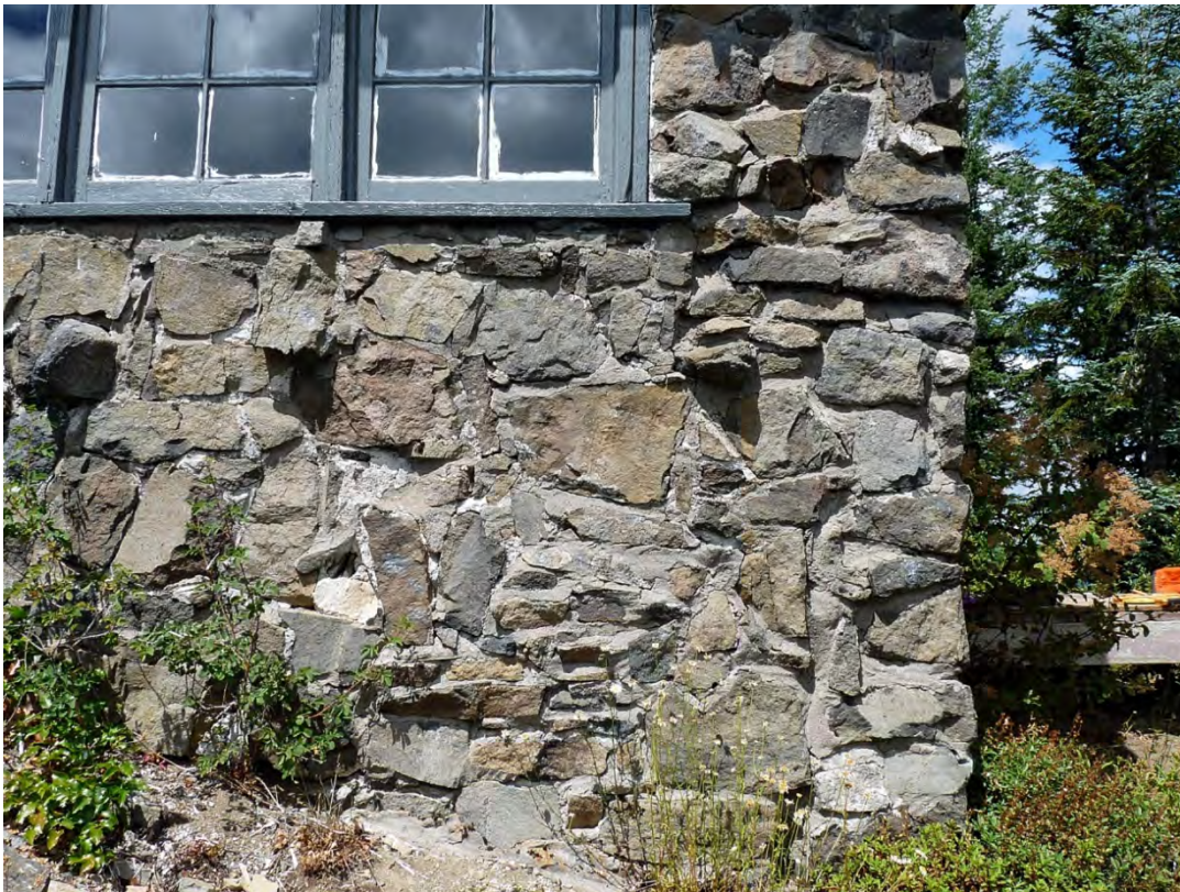
Figure 15. View of the local stone used in the construction of Pechuck Lookout.
