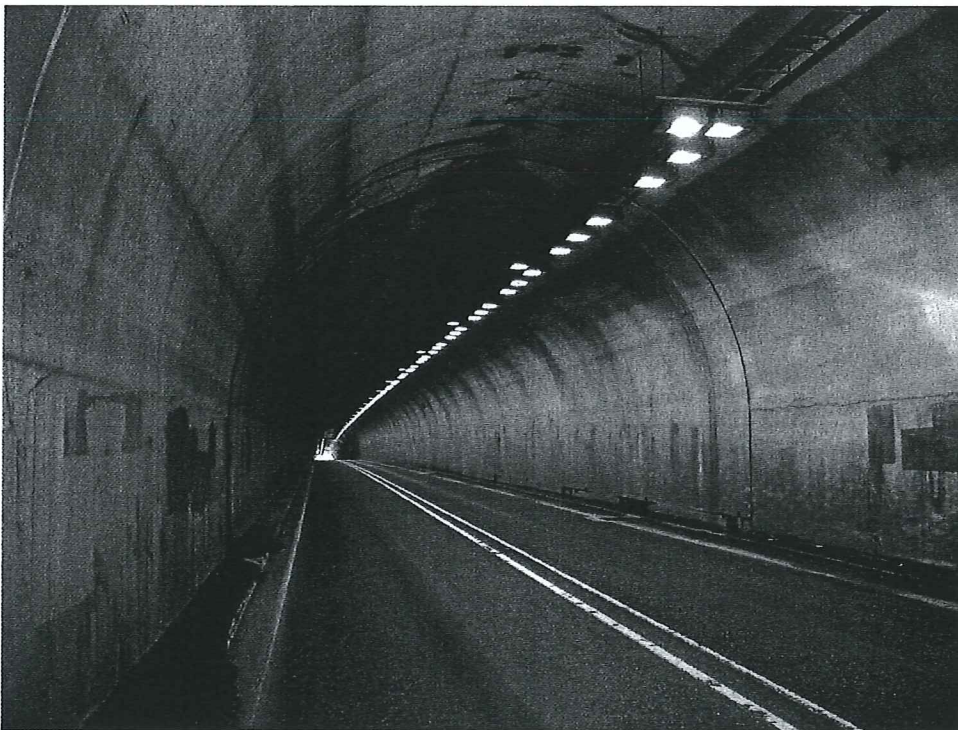
Suspended lighting system proposed for Salt Creek Tunnel. (Peterson Tunnel shown, system also installed in the Toothrock Tunnel)
