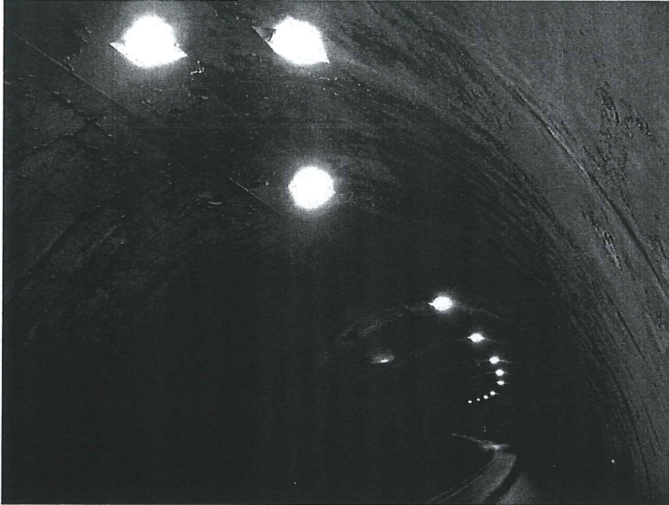
Existing lighting system looking east near center of tunnel.
