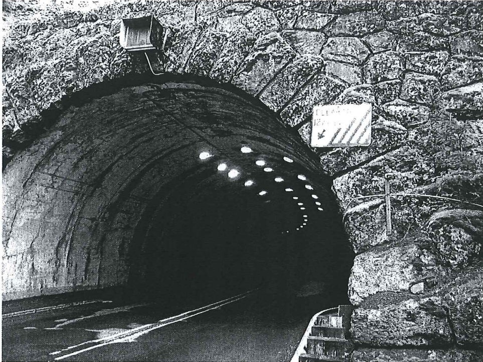
Existing lighting at west portal.
