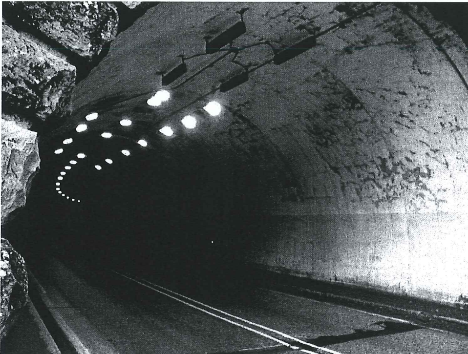
Existing lighting and de-icing system at east portal.
