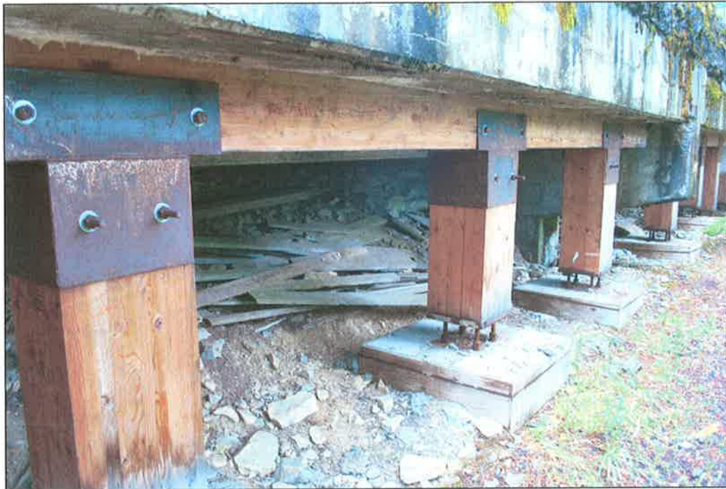
Figure 9: Half-viaduct shoring from 2006 to prevent potential failure
