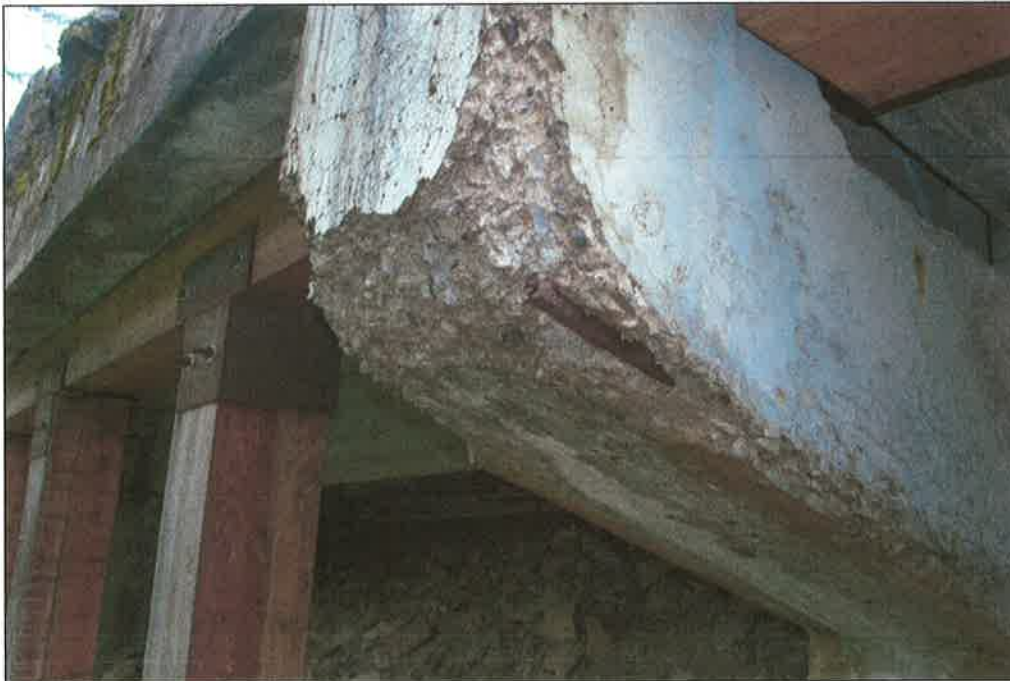
Figure 8: Spalling and section loss of half-viaduct concrete
