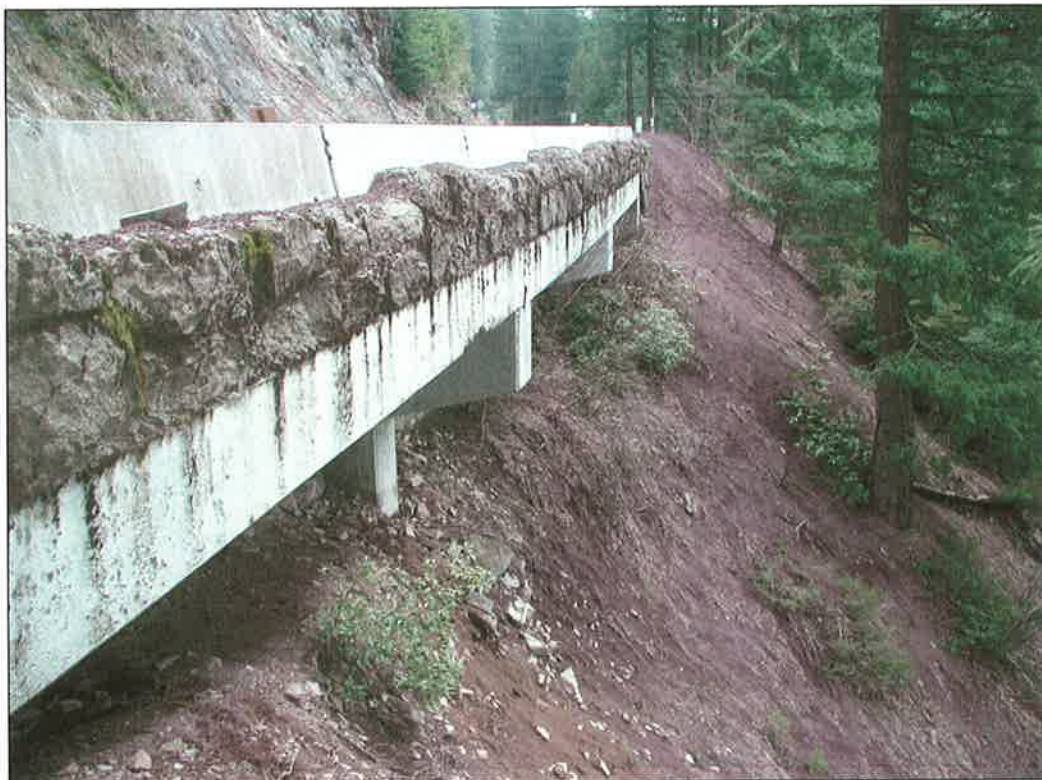
Figure 10: Crumbling masonry rock bridge rail parapet
