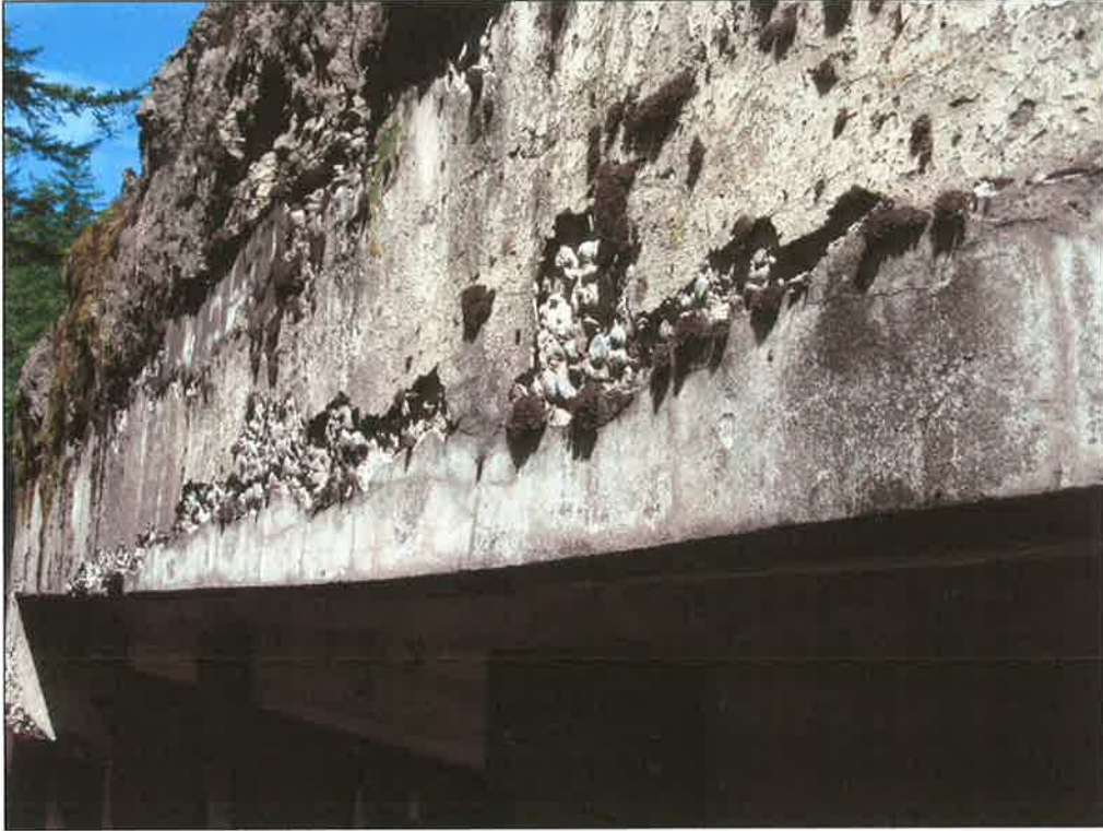
Figure 7: Severe deterioration (due to constant freeze/thaw) of half-viaduct
