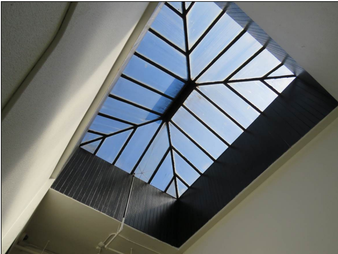
Photograph 16 of 20: OR_MultnomahCounty_GoldenWestHotel_0016 View of vaulted skylight over Golden West primary staircase, camera facing south.
