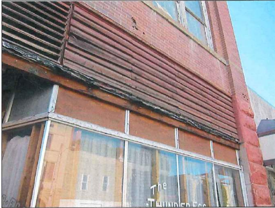
Photo 3 of 16: West (front) elevation showing south storefront and closed transoms, looking southeast July 2015
