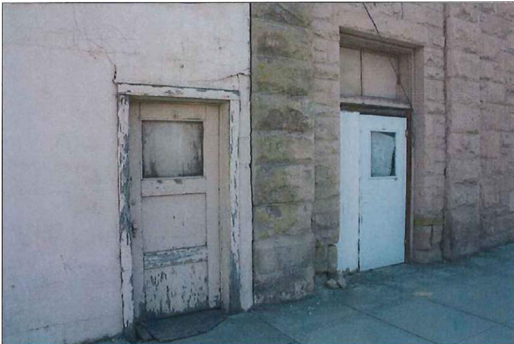
Photo 6 of 16: North elevation showing sandstone first story and the addition to the rear, looking south, July 2013
