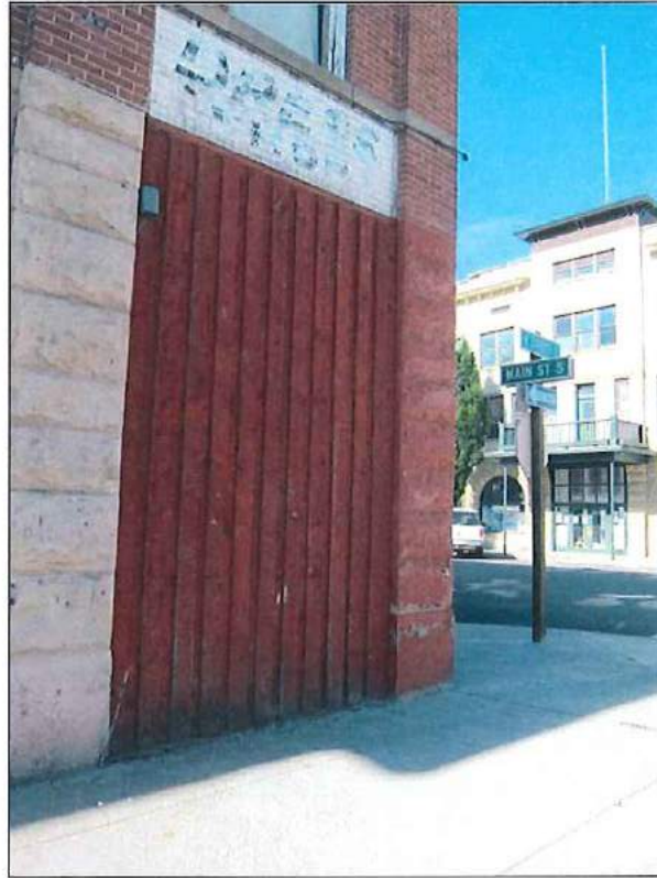
Photo 7 of 16: North elevation showing northwest corner with windows covered over and commercial sign above, looking southwest, July 2015
