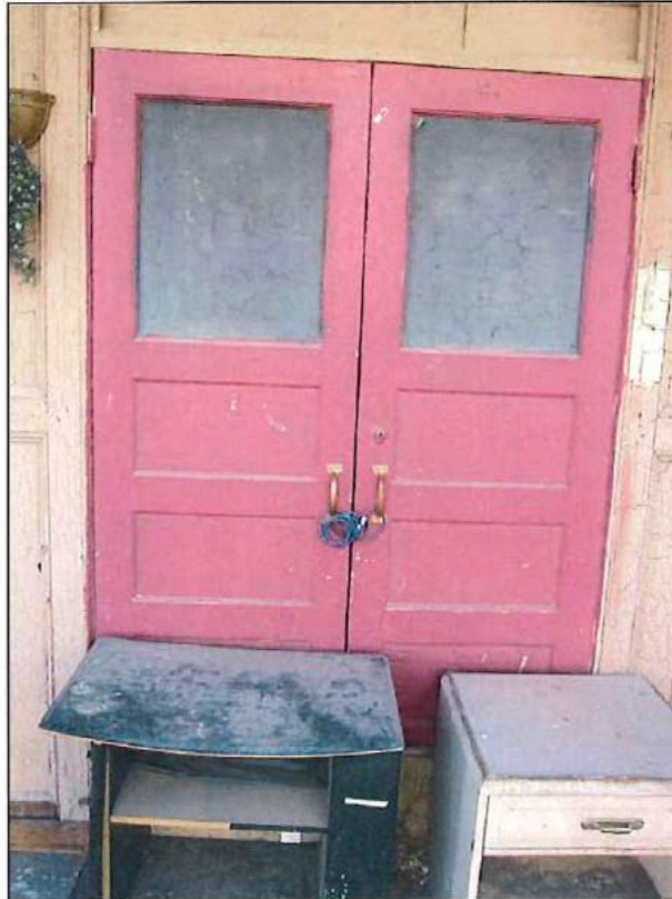
Photo 4 of 16: West (front) elevation showing the central set of double doors leading to second story, looking east, July 2013
