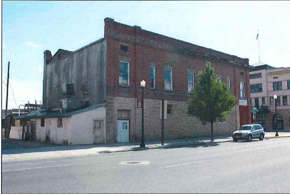
Photo 5 of 16: North elevation showing sandstone first story (right), addition to rear, and gunnite on east rear elevation (left), looking southwest, July 2013
