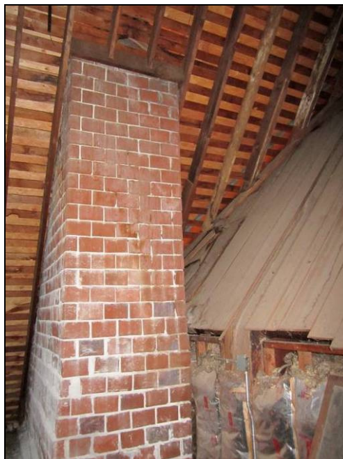
Photo 12 of 12: (OR_MultnomahCounty_RoseCityGolfClubhouse_0010) Attic. The room is unused, but features the original skip sheathing for the original shake roof and the original brick chimney.
