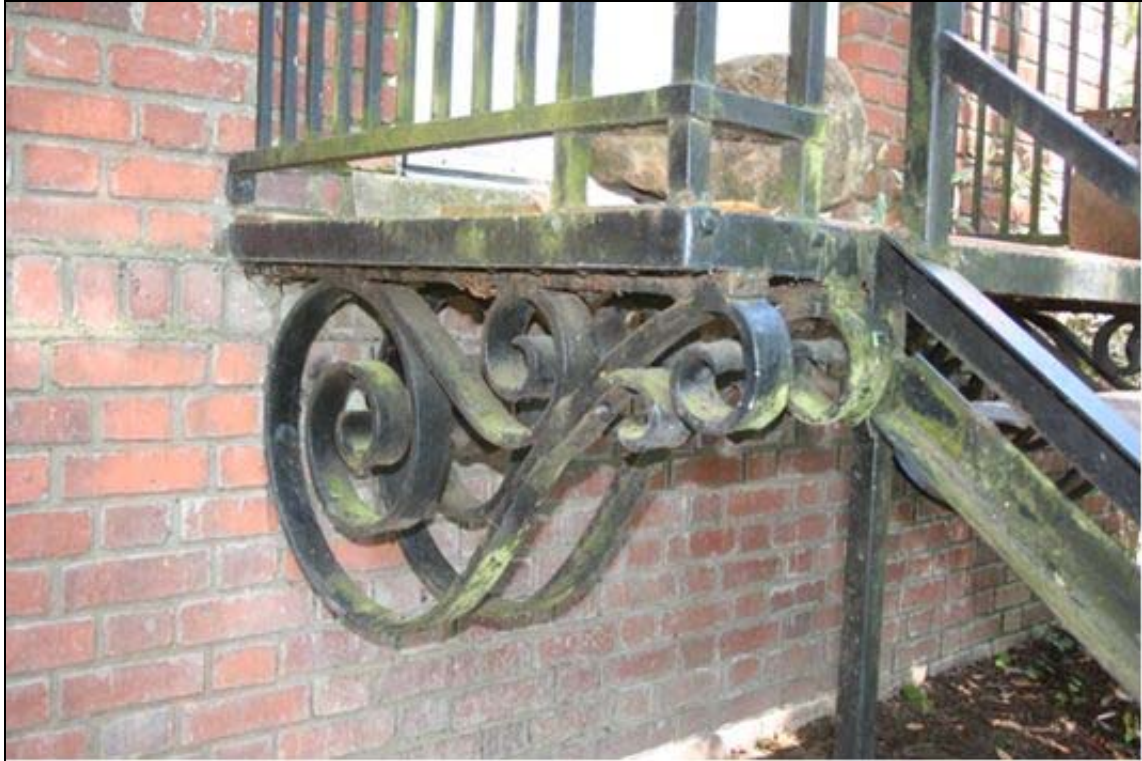
Photo 9 of 16: OR_DouglasCounty_ORStateSoldiersHomeHospital_0009 Detail of iron stairs bracket under west façade entrance stairway, looking southeast
