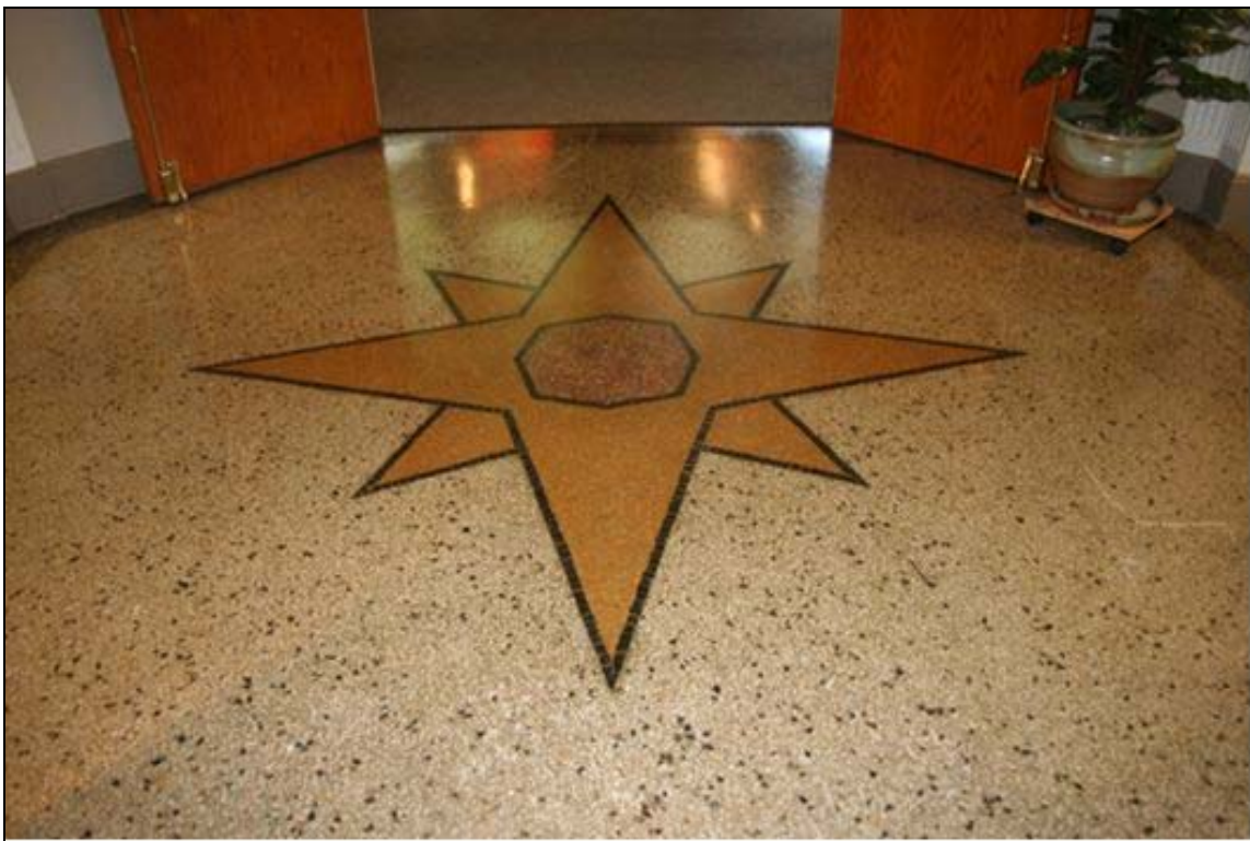
Photo 14 of 16: OR_DouglasCounty_ORStateSoldiersHomeHospital _0014 Detail of compass rose pattern in terrazzo floor at the intersection of the entrance and central halls
