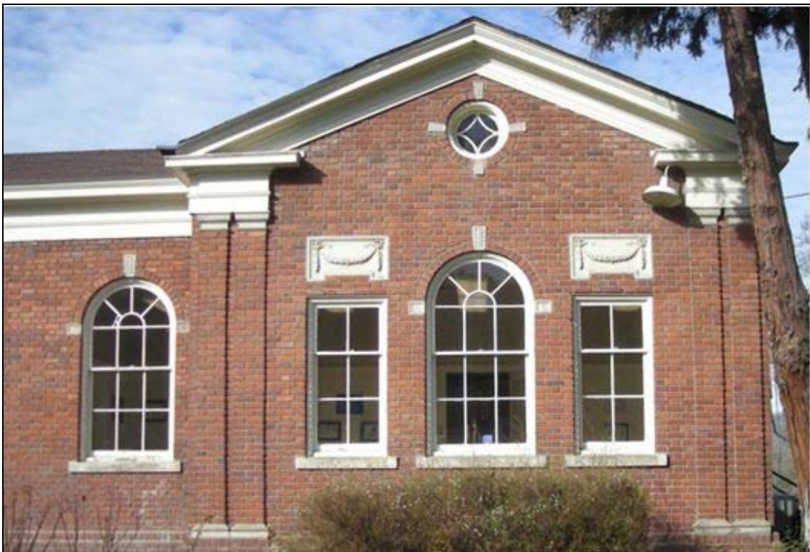
Photo 8 of 16: OR_DouglasCounty_ORStateSoldiersHomeHospital _0008 East wing of the south façade, detail of decorative details, looking north
