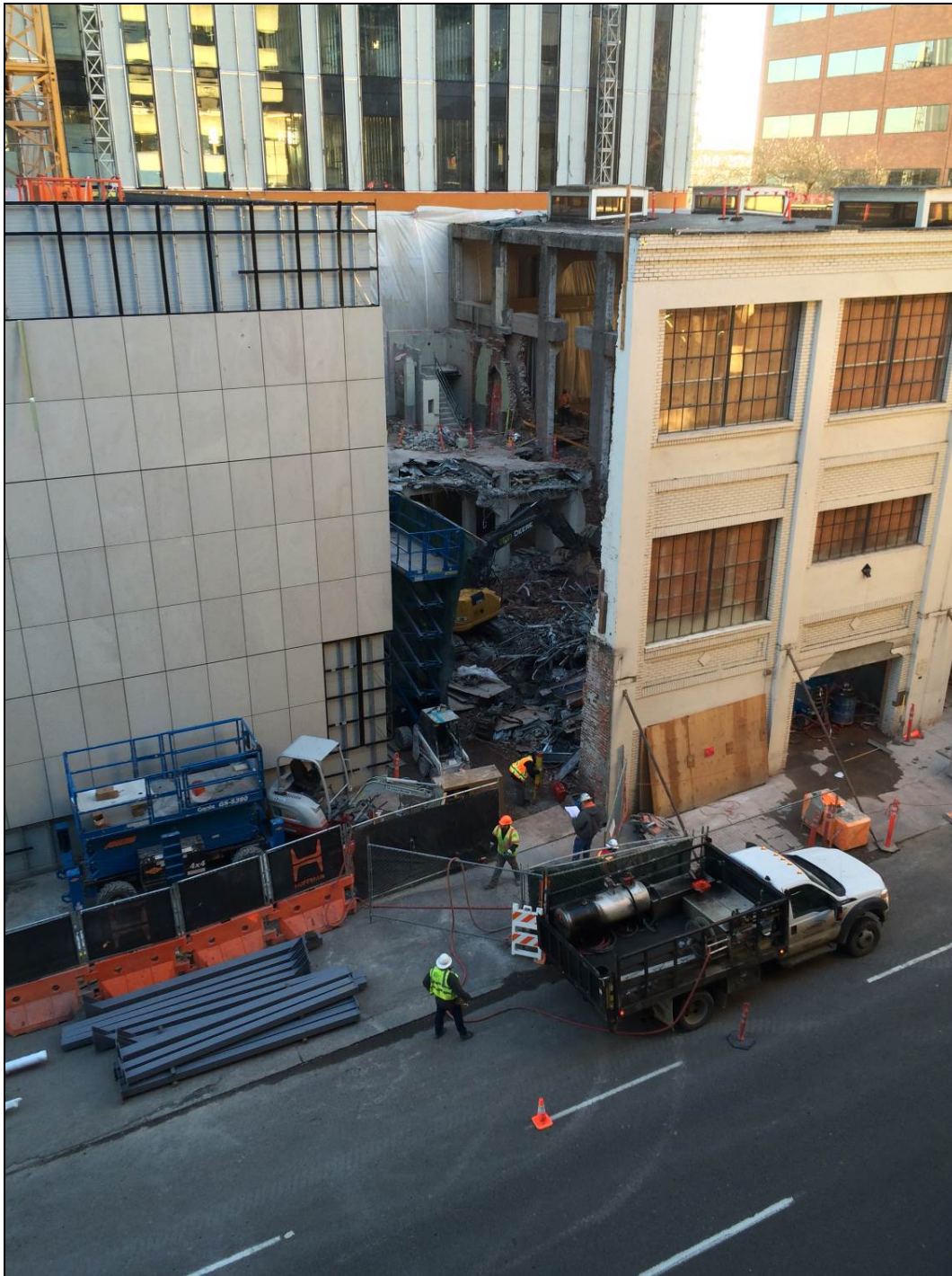
Figure 16: Photograph of demolition activity removing all interior fabric of 1925 addition, looking southeast. January 22, 2019.
