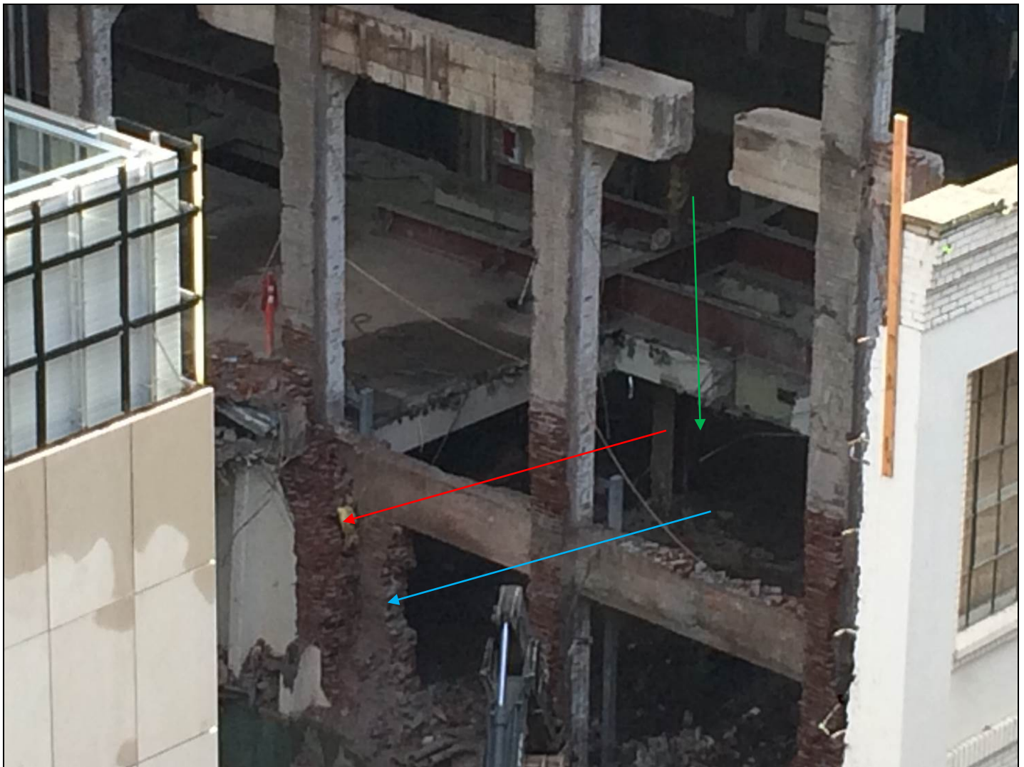
Figure 17: Detail photograph of demolition activity, showing removal of brick masonry walls of 1925 addition (red arrow), intervening brickwork between structural columns of 1909 building (blue arrow), interior room divisions, floors (green arrow) as well as structural beams, looking southeast. January 22, 2019.
