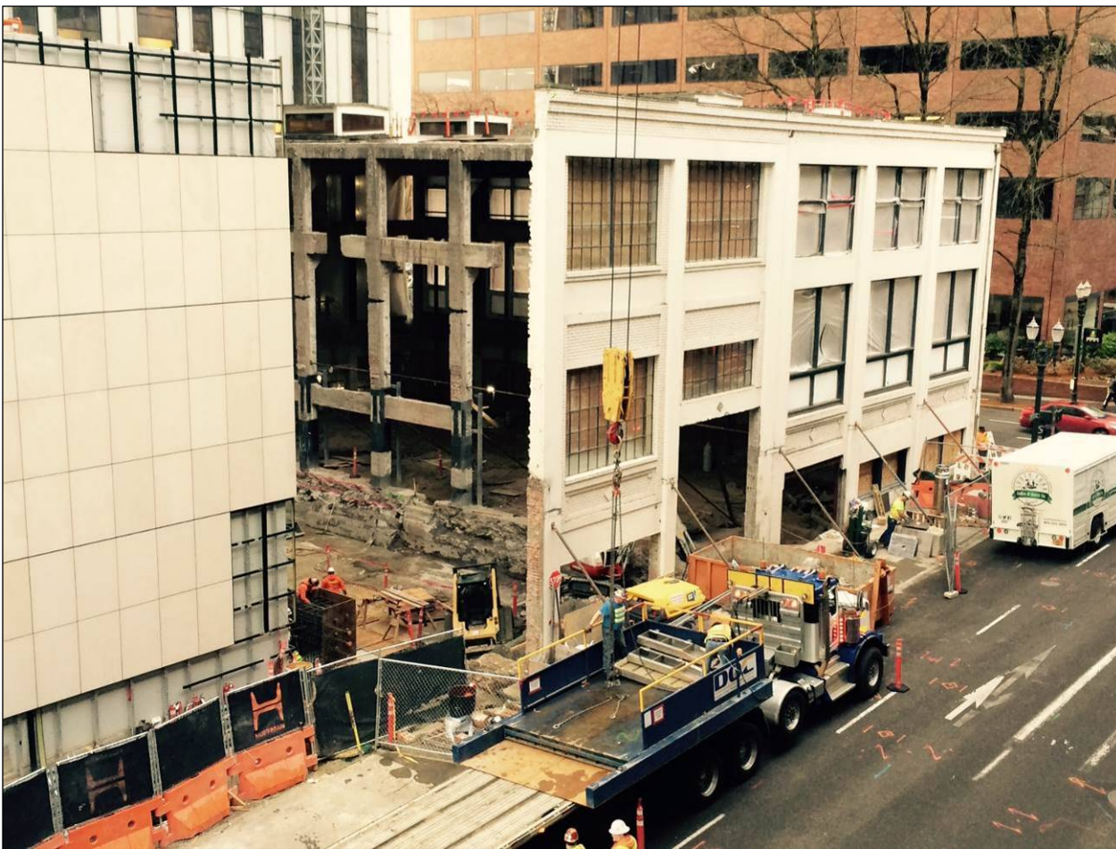
Figure 20: February 2019 view of Jefferson Station. All interior components of the 1925 addition have been removed to expose the basement level. The basement level was subsequently infilled up to the first floor in April 2019.
