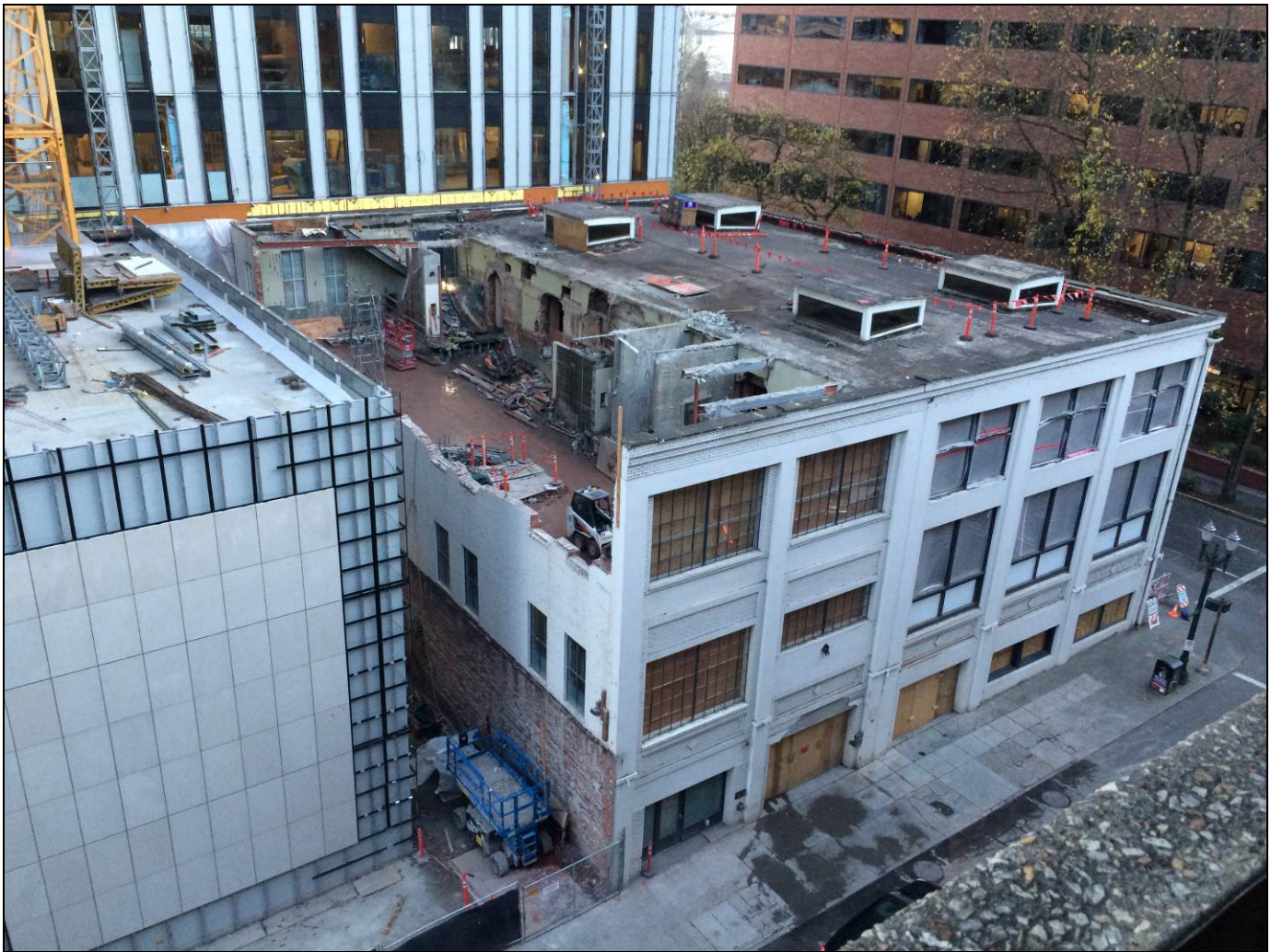
Figure 13: Photograph of demolition activity, looking southeast. December 6, 2018. Note the presence of reinforced concrete interior room subdivisions present on the partially demolished third floor.
