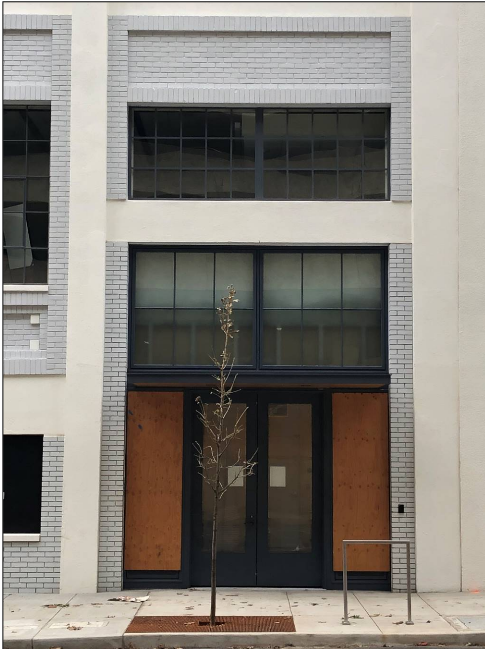
Photo 4 of 6: OR_MultnomahCounty_JeffersonSubstation_0004 Photograph of west entrance with boarded up glazed single pane sidelights, glazed Pella doors, and oversized pane transom. October 15, 2020.
