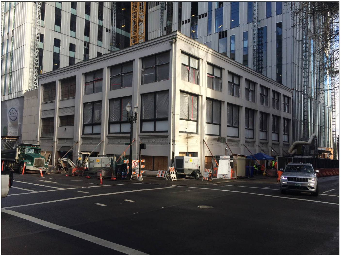
Figure 21: Photograph of west and south elevations. The windows have been removed from the 1909 part of the building. Original windows appear intact on 1925 addition. January 22, 2019.
