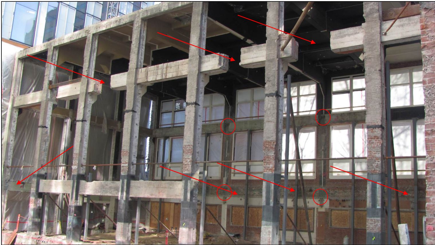
Figure 18: Photograph of interior of 1909 Building. Red arrows show complete or total loss of lateral concrete supports. Circles indicate ghosts of 10 haunched transverse beams removed during demolition activities in 1909 building (Note: some of the ghosts are hidden behind the vertical supports in foreground – a total of twelve were removed). All voids between exterior structural columns and beams were formerly filled with five-to-one common bond brickwork. The photograph also confirms the loss of all interior reinforced concrete floors. Five haunched beams remain in the upper floor to carry the weight of the roof. March 24, 2019.
