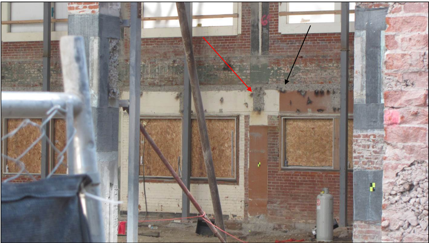
Figure 19: Detail view of the interior of the south wall, looking south. Black arrow points to ghost of reinforced concrete floor removed during 2018-2019 demolition activities. Red arrow points to ghost of former transverse beam. March 24, 2019.
