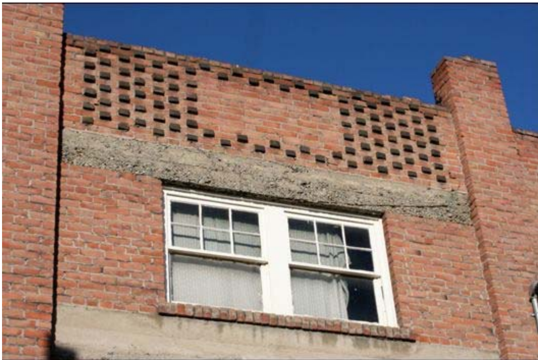
Photo 6 of 16: OR_WallowaCounty_EnterpriseIOOFHall_DowntownEnterpriseMPD_0006 Brick detail on the west corner of the south façade, looking north.
