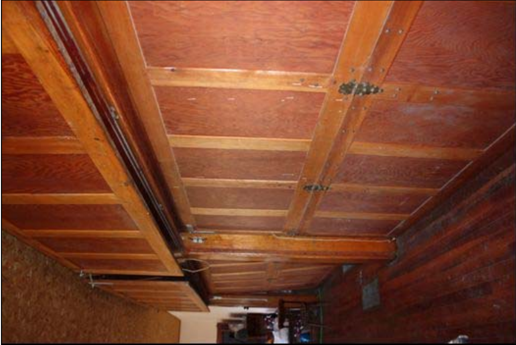
Photo 11 of 16: OR_WallowaCounty_EnterpriseIOOFHall_DowntownEnterpriseMPD_0011 Detail of the wood partition panel doors in the clubroom, looking southwest.
