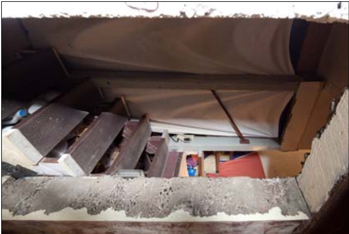
14 of 14: OR_MultnomahCounty_GeorgeWandHettyABowersHouse_0014 Stair to basement and concrete wall opening, camera facing northeast.
